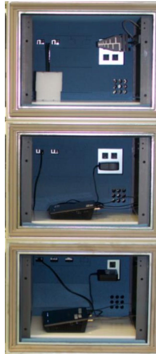
Alternative cabling with no splitter and with the iGen interference generator/monitor
