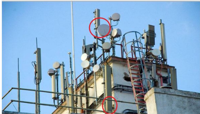
Figure 1 – example of antennas close to metal infrastructure
