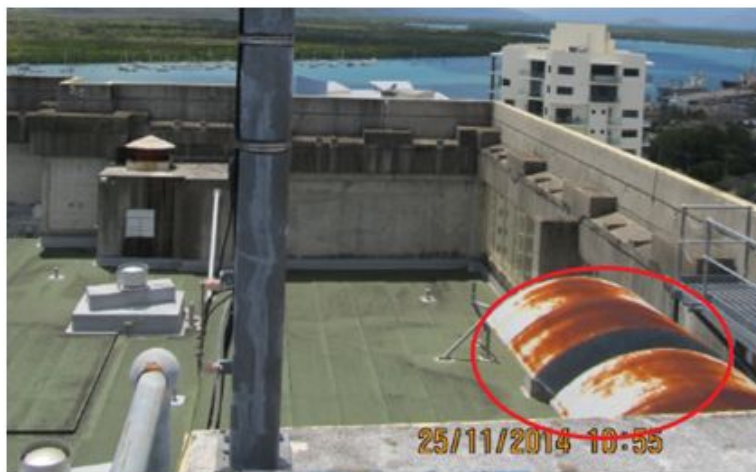
Figure 2 – rooftop cell site with a nearby rusty roof
